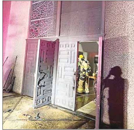
Damaged the sanctuary, historic front doors and stained glass windows of Congregation Beth Israel in Austin, TX
